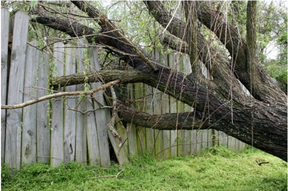
Figure 5, an image of a fence which a tree has fallen onto
